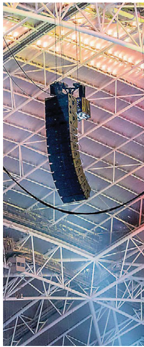
Two Nexo Universal Amp Racks (NUAR) were flown behind each array to reduce cabling length and weight
