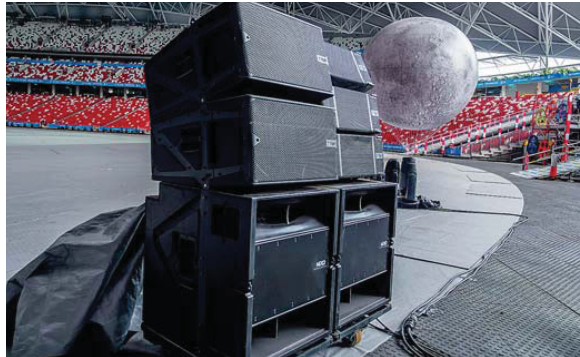
Seats in the first tier were covered by ground-stacks with three M28 mains, two B112 bass enclosures and two S118 subs
