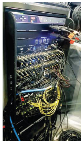
A dual redundant Optocore fibre ring was provided for networking
