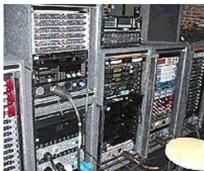
Outboard racks, monitor world
